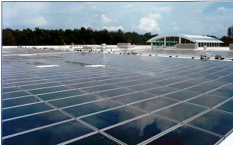
Photo 5 - The EPA's Computer Center handles a massive quantity of data processing equipment. The output from the solar collectors offsets approximately 5% of the building's energy consumption, which is estimated to be approximately twice that of a conventional office building of equivalent size, due to the large demand from data processing equipment. Photo courtesy of the EPA.
