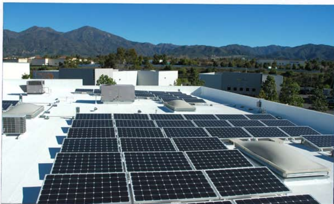
Photo 1 – One solar installation company that has embraced the marriage of solar panels and cool roofs is Advanced Powering Services, Inc., of Rancho Santa Margarita, CA. The company has installed a cool roof/solar panel beta test site on the roof of an industrial building. Photo courtesy of Coat'N'Cool.
